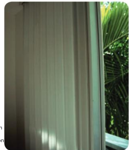
Figure 8.21 (a and b) Steel shutters for hurricane management at the Casuarina Hotel, Barbados
