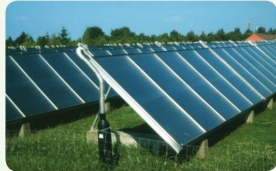
Figure 4.23 Solar panels, Aero Island, Denmark
